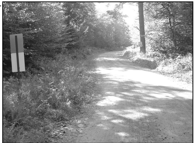
Before: A photo of Cove Way in the Branch Lake Watershed prior to road work. Notice the lack of proper ditching and extensive plant growth on the left side of the road.
