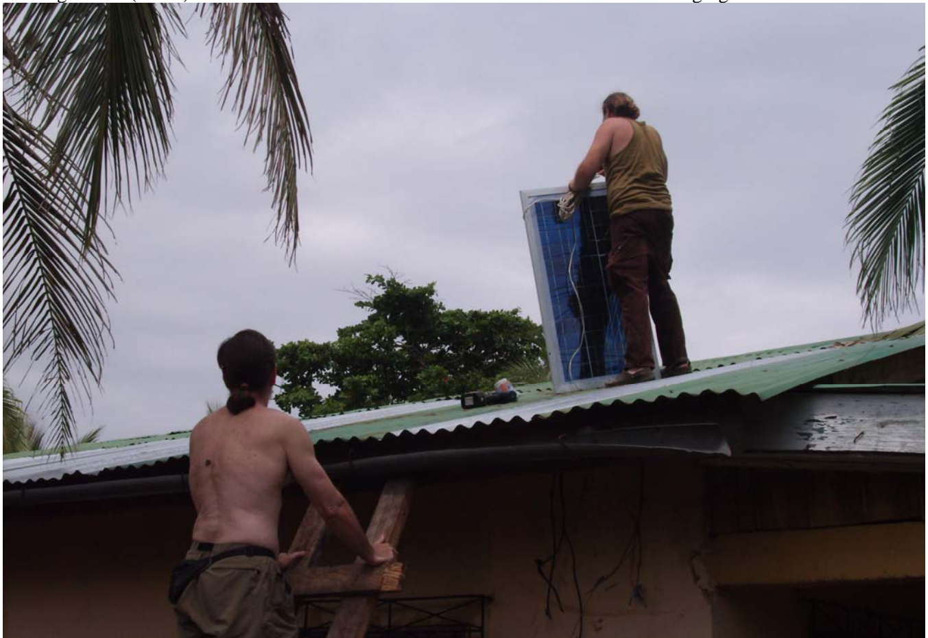
Installing the 60 watt PV module we had just finished building, onto the roof of Cody's new home.
