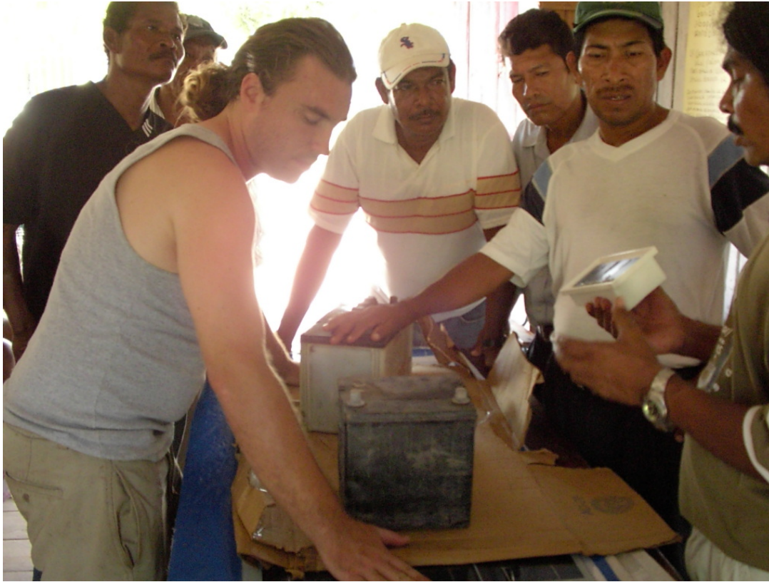
Using old car batteries as weights to laminate the 60 watt PV module.
